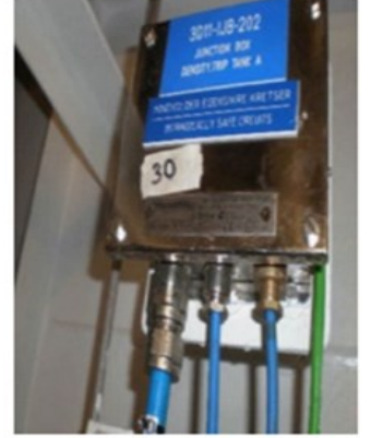
Improper Cable Gland Installation/Modification
