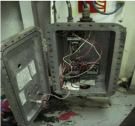
Improperly Modified & Maintained Certified Safe Junction Box
